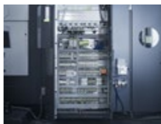
Climatized electric cabinet with easy access.
